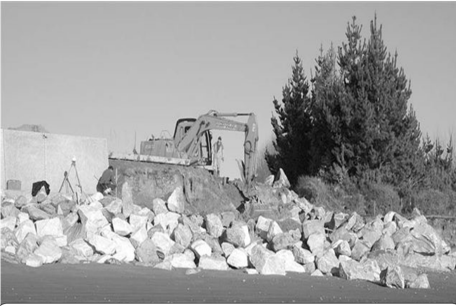
Workmen with help from an excavator install part of a controversial concrete wall on a beachfront property owned by a company called Harlequin Trading. The northern end of the wall adjoins the part of the Old Mill Walkway most eroded by recent storms
