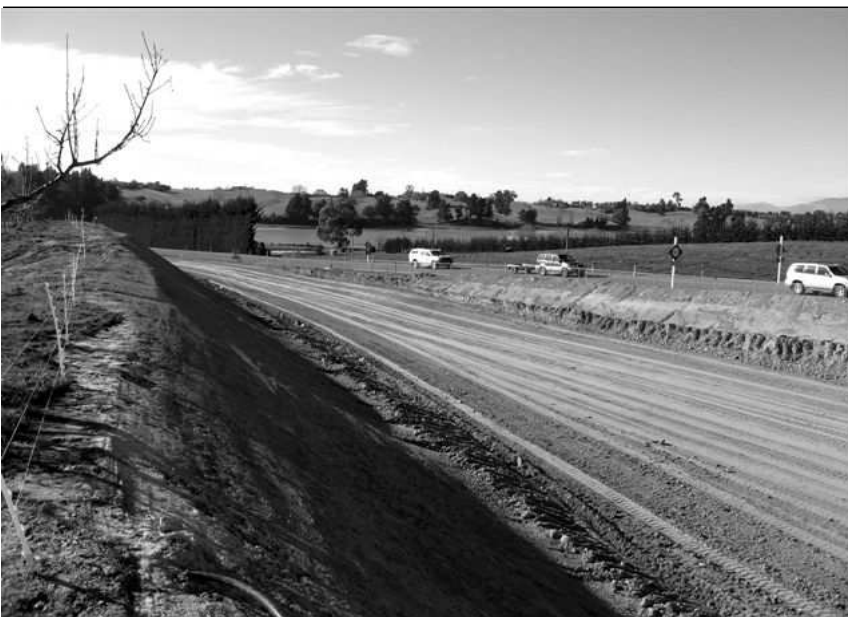
The new roadbed beside SH60 from Apple Valley Road looking towards the estuary.
